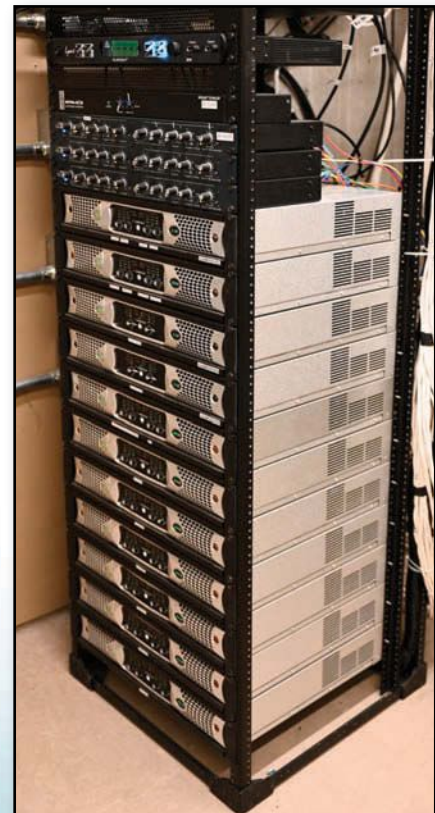
The equipment rack
